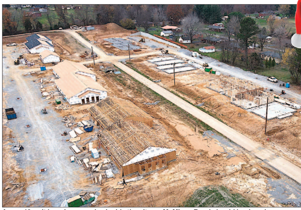
A new 48-unit housing complex inside the city on McMican Road should be done by summer.
